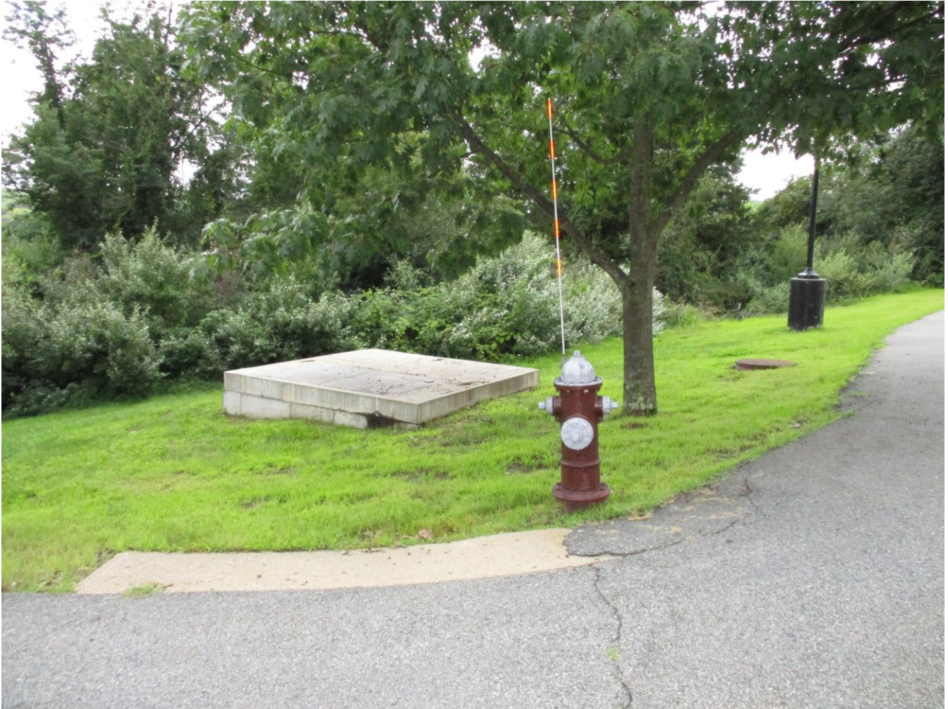
Water system vault for LHT and Darymple House
