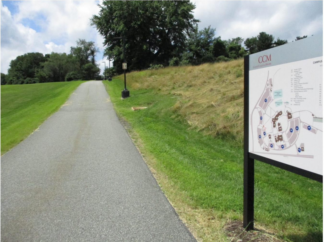
Electrical vault heading from Lot 1
